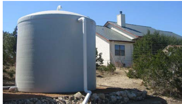
Wet conveyance system example
