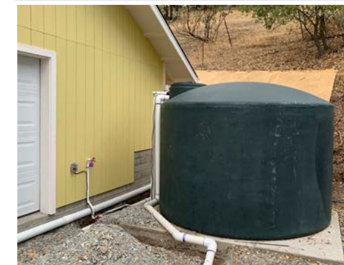
Example of a polyethylene or polypropylene (plastic) rainwater tank. They are the most common material used for residential rainwater systems and are available in various sizes. Source: Watershed Progressive
