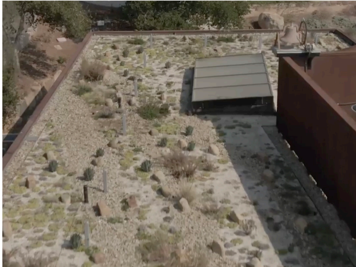
Image 1: Green Roof at the Thacher School in Ojai, California (Source: Watershed Progressive)
