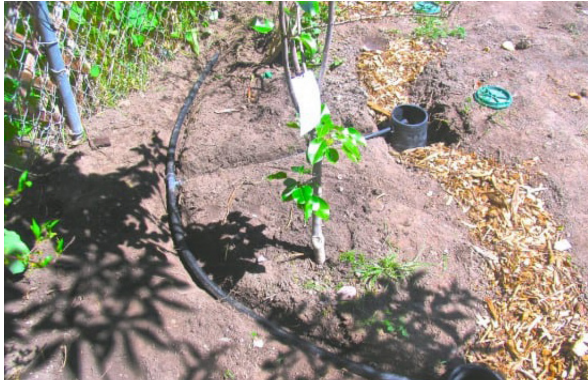
Image 1: A greywater system installation showing mulch basins. (Source: GreyWaterAction.org)
