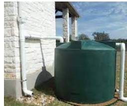
Example rain tank
